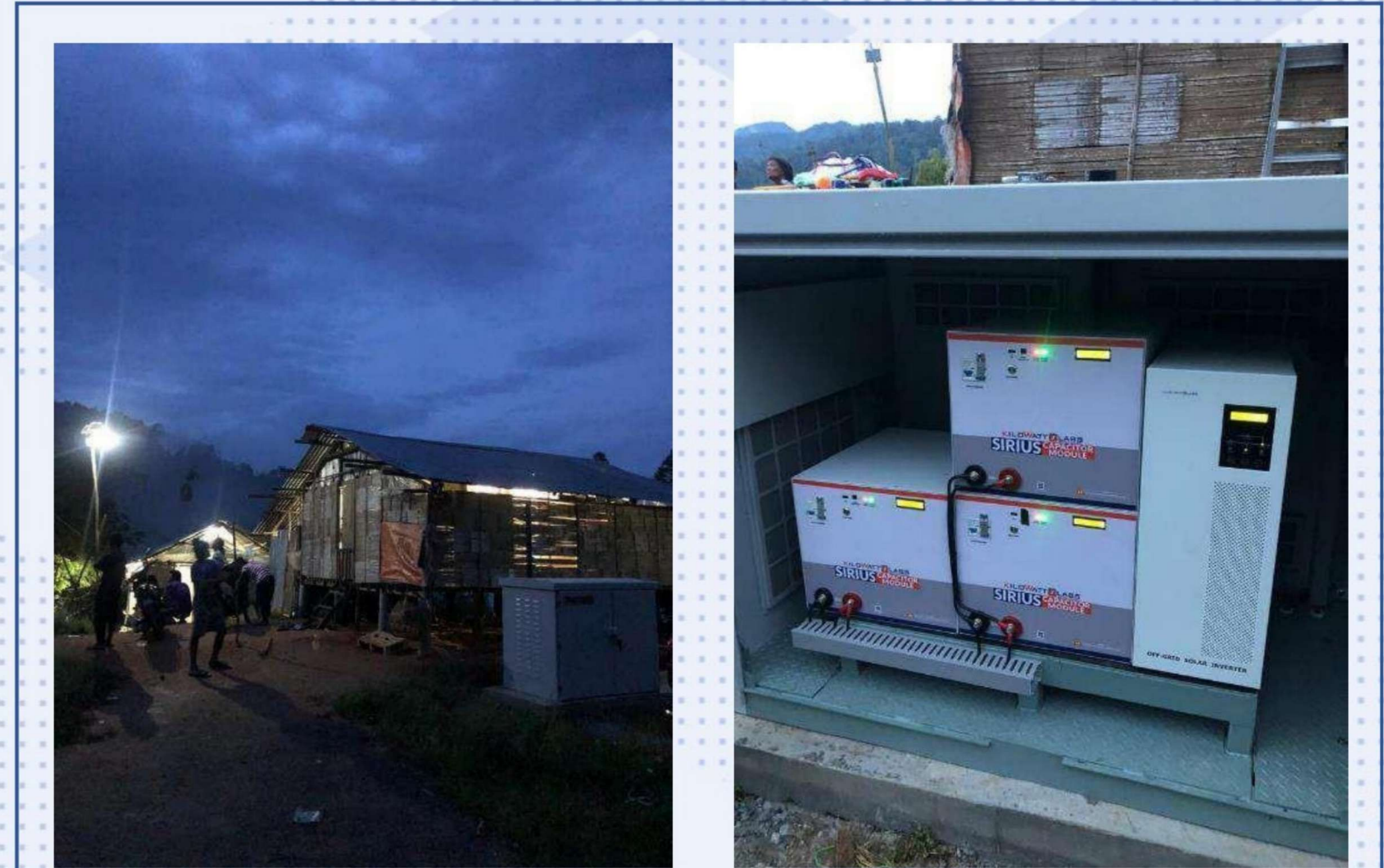
Remote Microgrid Site – Malaysia
