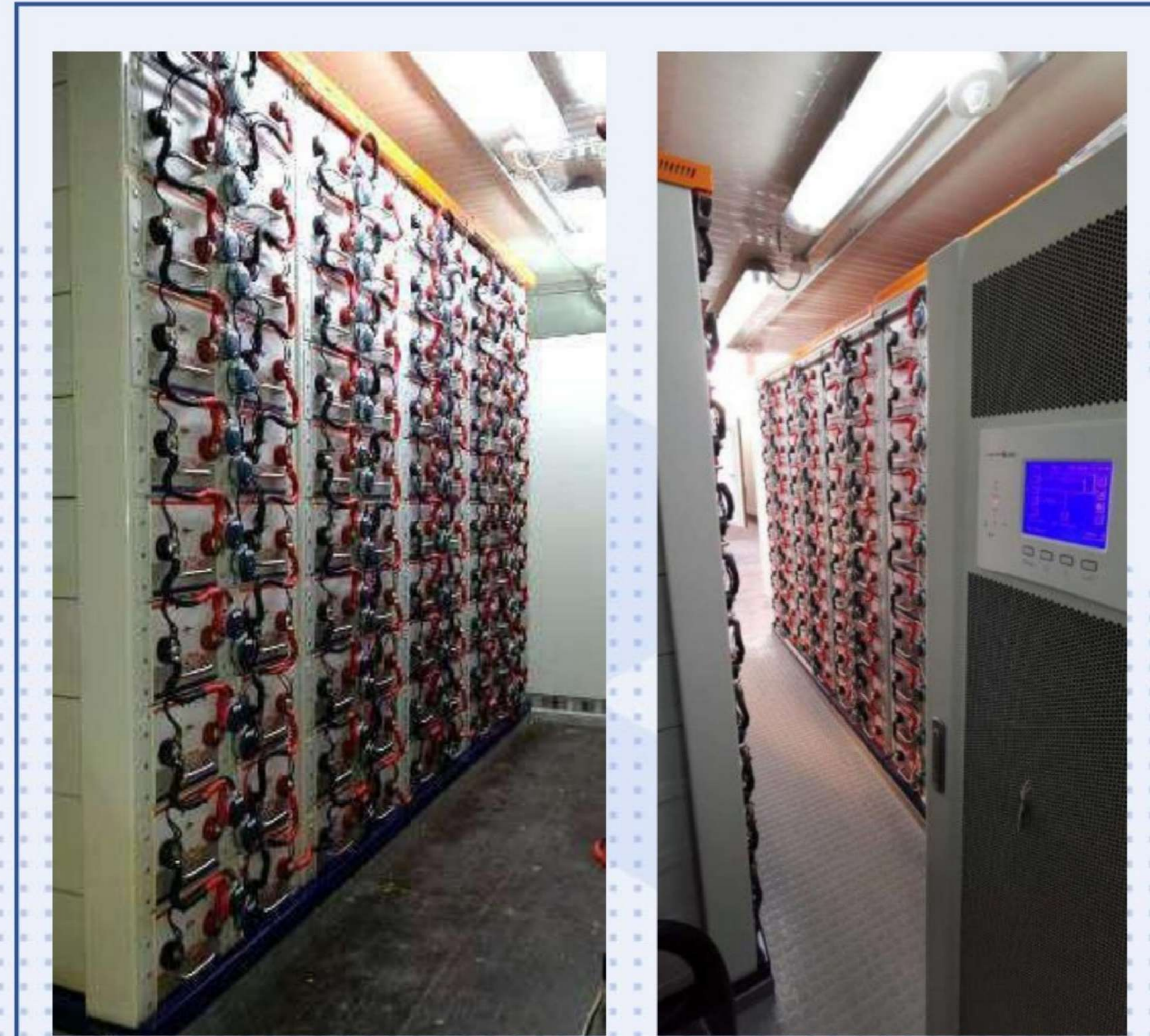
Containerised Microgrid – USA
