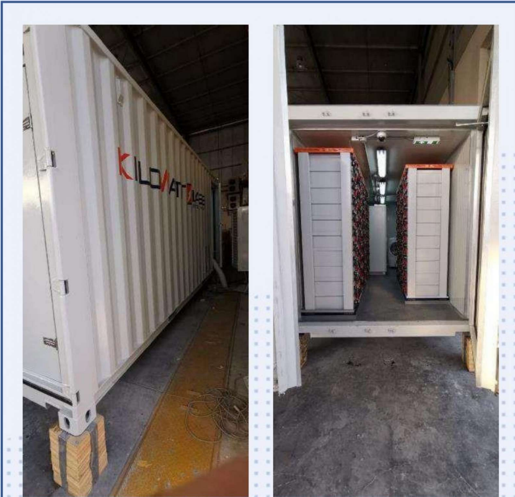
Containerised Microgrid – Kenya
